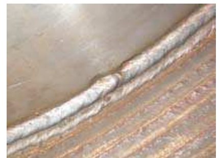
b) membrane weld joint lack of fusion during welding and cut up weld joint
