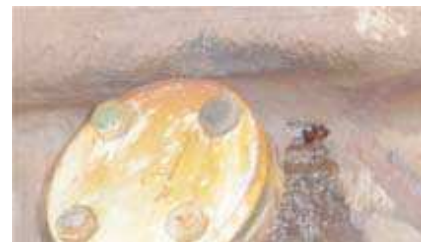
b) another shell penetration damage
