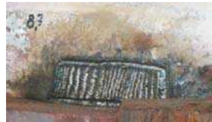
a) welded shell penetration damage
