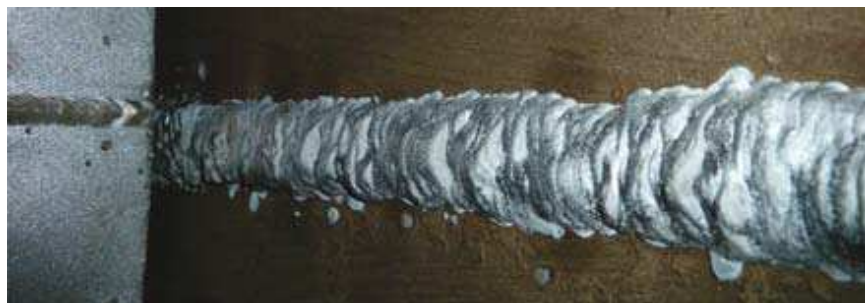
d) repair overlay of the base welding joint. Done manually by arc welding with a coated electrode – spits on base metal, bad weld joint geometry and large beads
