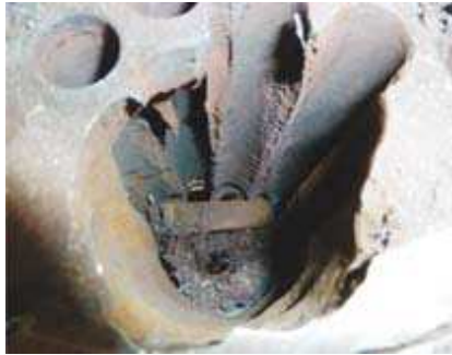
d) tube sheet damage
