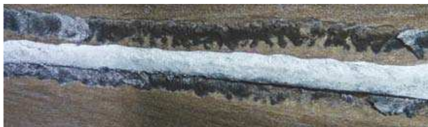
c) overlay welding joints completely destroyed by corrosion caused additional thinning of the liner with depth of 2 mm. Wrong welding consumables were used.
