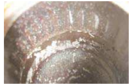
Picture 4.1 – Pitting corrosion on inner surface of heat exchanging tubes The pitting was the result of the wrong welding parameters used at fabrication stage.
