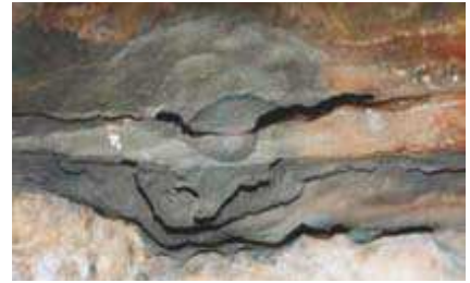
b) Corrosion damage of the shell with the depth reaching 25 mm
