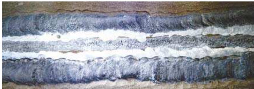
a) thinning in HAZ in repair welding joints with depth up to 1 mm – high amperage during the welding, black weld bead with cavities – insufficient protection of the welding groove
