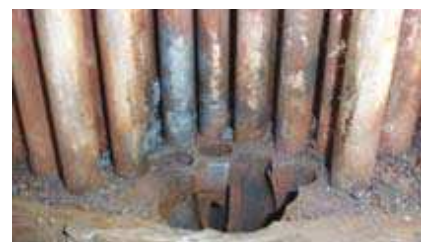
c) tube sheet damage revealed after shell and tubes were dismantled
